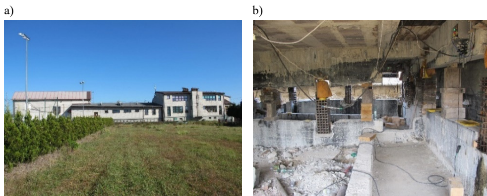
Fig. 5. School building: a) view from the east, b) object during rectification – jacks built into the walls ( own research )
