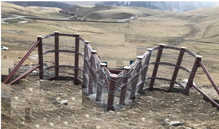
Fig. 6. An overview of an innovative snow avalanche construction Georgian Military Road in Kobi-Gudauri alpine zone (2238 m above sea level) ( own foto )
