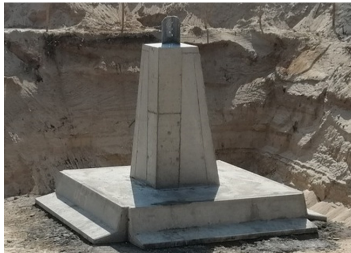
Fig. 1. View of innovative monolithic-prefabricated foundations at the Piła-Krzewina-Plewiska tower site (Enprom Report, 2018)
